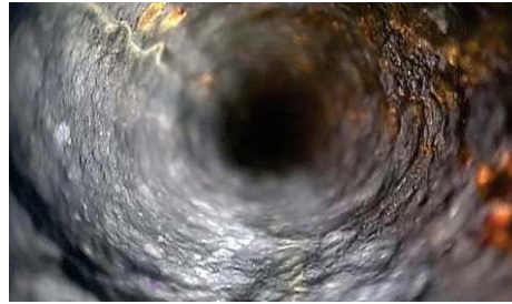
Real-Life Problem 2 Corrosion of Piping
